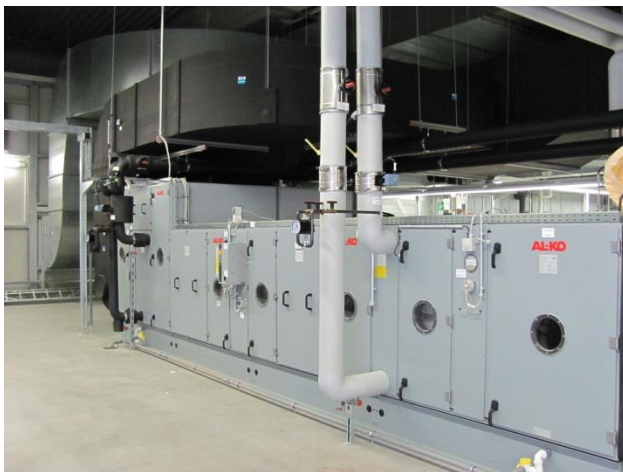
Figure 9: Tunnel Air Handling Unit.
